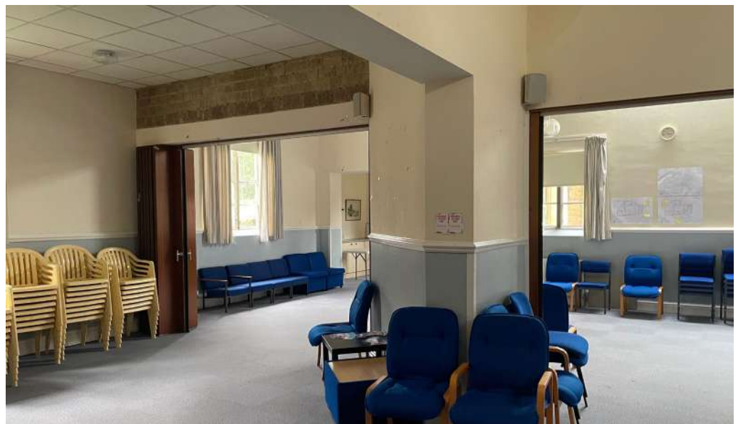
Figures 4.12 and 4.13 - internal photographs showing the beams inserted in the 1990's, when the walls were removed
